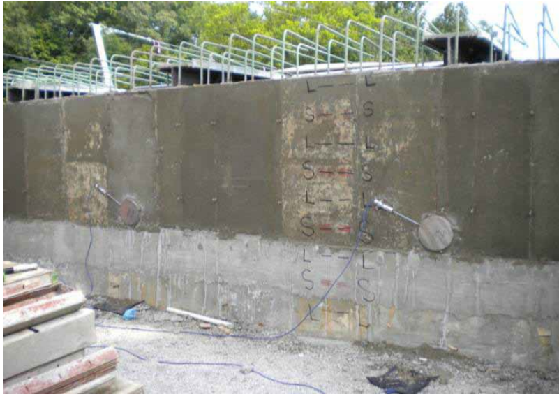
Figure 7. Pressure cells behind the back wall on Tiffin River Bridge (Adam et al., 2011)
