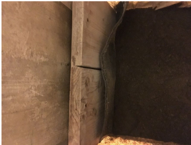
Figure 42. Gap between concrete wall and wrap-around geosynthetic
